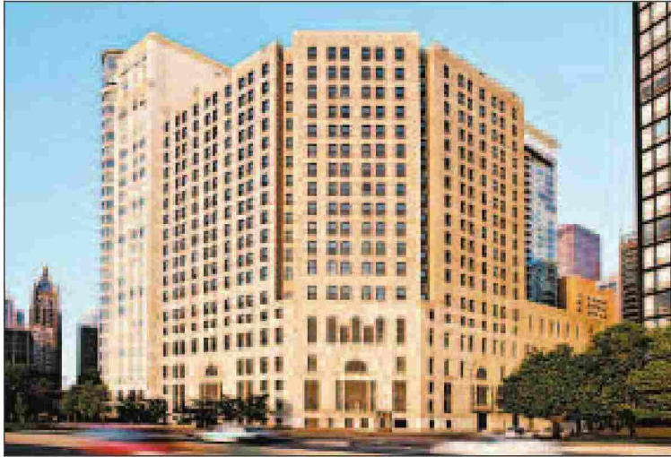
Work is under way at 850 N. Lake Shore Drive. The former Lake Shore Athletic Club is being converted into a retirement building.
